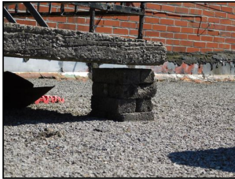
(Concrete) The upper balcony has sloped and cracked due to settlement and or support under an area. Important repairs will be needed.
