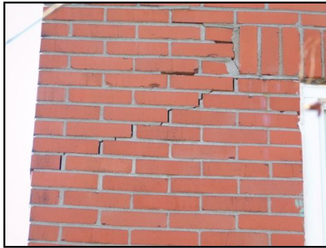
(Step crack active) Cracking visible in brick exterior walls appeared to be consistent caused by differential settling of soil and/or the foundation.
