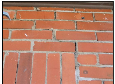
All cracks and openings on exterior coverings should be sealed and repaired to prevent water infiltration and further damages.
