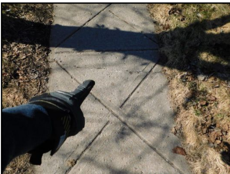
Common cracks and heaved/settled areas observed.
