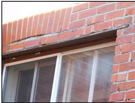
Slight sag observed on the lintel
