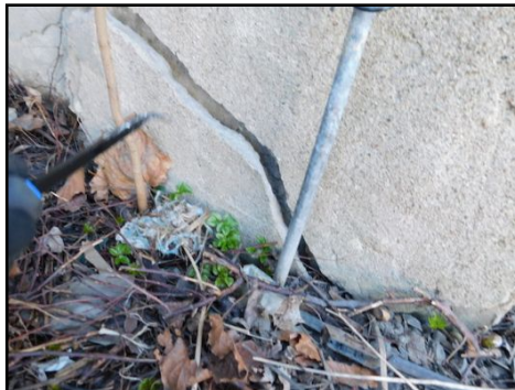
Parge crack, foundation crack was not observed. Limited visibility
