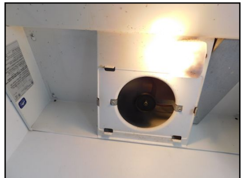
Hood fan: Missing screen, installing one is recommended to enhance safety.
