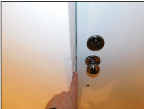
Front door rubs on the wall
