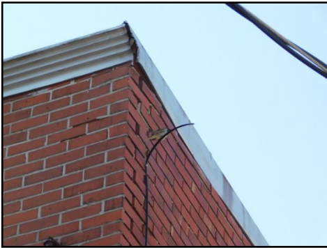
Corrosion, deterioration, openings and poor condition of the caulking was noted on the flashing. This condition can easily lead to water infiltration within the walls. Corrections required by a qualified roofing contractor.
