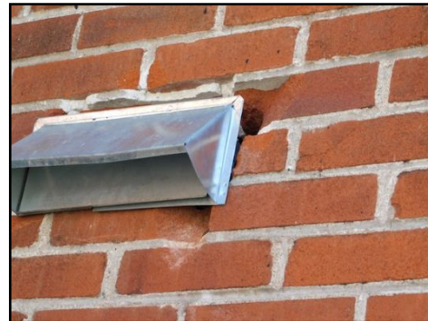
Note: It is recommended to caulk around all fixtures and exterior penetrations. Leaving areas of penetration with missing, improper or defective caulk could result in leakage, rot and/or even the possibility of mould formation. Regular caulk of all potential leakage areas should improve these conditions.
