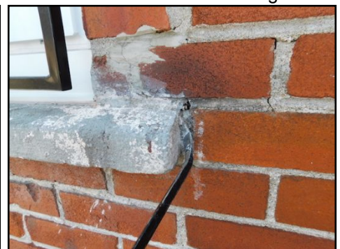
(Openings at the edges of the sill joints) Cracks/openings observed at the edges of the sill joints. This condition can lead to water infiltration and deteriorate the masonry materials below the windows in a faster speed. Repairs and corrections required on a regular basis to prevent degradation and spalling.
