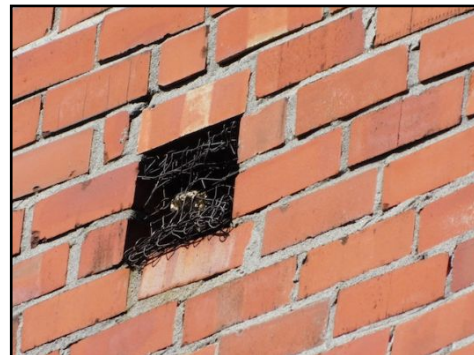
Damaged screen, possibility from animal, and may have entered. Verify and repair screen
