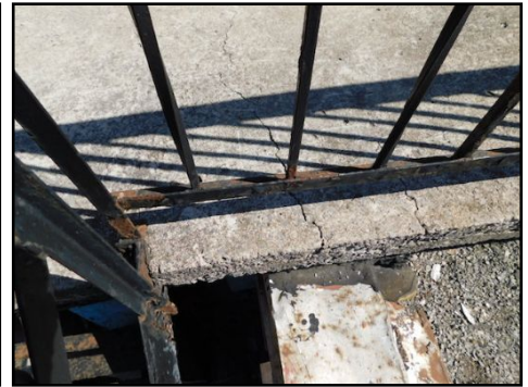
(Concrete) The upper balcony has sloped and cracked due to settlement and or support under an area. Important repairs will be needed.
