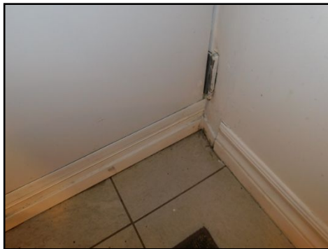
Appears to be previous water stains/infiltration/ Dry at the time. Monitor the area and repair as needed.
