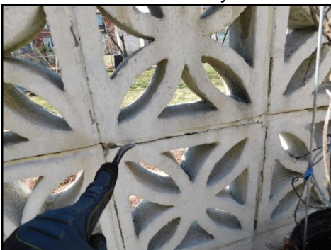
Guardrail is loose/detaching. Important repair needed. (Also a safety hazard)
