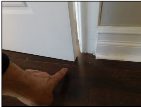
Door rubs on the floor
