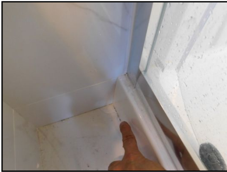
Standing shower and surrounding: Prefabricated fiberglass. Leaks noted (on both edges of the shower surrounding) at the time of the inspection. Repair required to prevent water damage.
