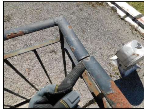
Guard rails cracked open. Replacement needed.
