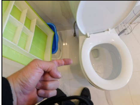
Toilet: Loose toilet was observed. This condition could result leakage and damages to the subfloor and other components. Corrections are required.
