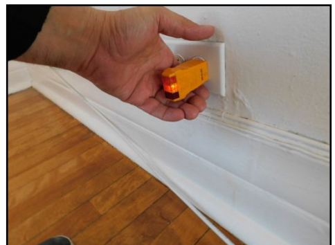
Electrical: - Outlets are not grounded (Also see main electrical).
