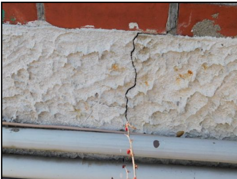
Foundation crack to be verified by foundation specialist and repair as needed
