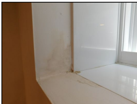
Walls and ceilings: Drywall. Previous signs of water damage/infiltration observed on the window sill sill. No moisture detected at the time of inspection. Verified with a moisture meter.
