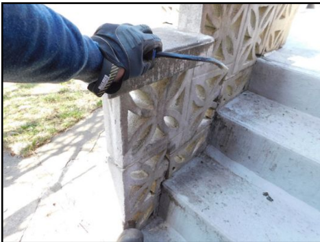
Loose handrail noted with the lower concrete block style handrail. This is a safety hazard. Corrections required to enhance safety.
