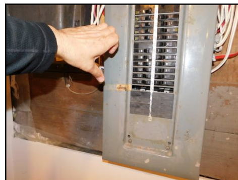
This is the older type electrical panel and it may no longer be acceptable by some insurance companies. It is recommended to consult with your insurance company for all rules and regulations that they may have regarding this situation.
