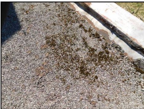
Moss/fungi growth observed. This is often a sign of high level of humidity in the attic area and on the wooden structure, however this was not verifiable due to limited access.
