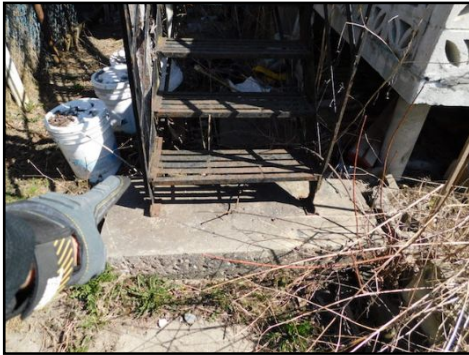
Uneven steps were observed, these are a trip hazard.
