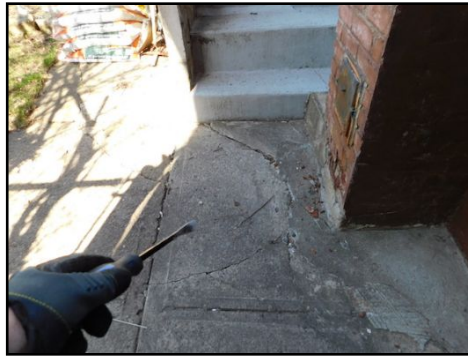
Uneven walkways were observed, this is a trip hazard
