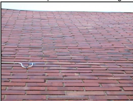
(Brick detachment) Visible brick detachment, and some appear to be bowing outwards was noted on upper portion of the building. This is often associated with water infiltration and freezing and is usually caused by improper flashing of the roof. Repairs and corrections required by a qualified contractor to prevent further damages.
