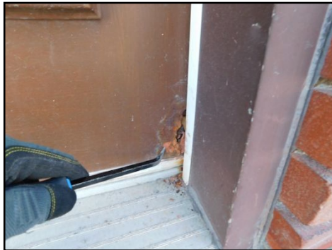
Corrosion, wear and tear observed. Recommend replacing the door (Prevent further rust, perforation and possible water infiltration due to rust)
