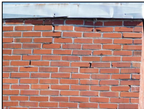
All cracks and openings on exterior coverings should be sealed and repaired to prevent water infiltration and further damages.
