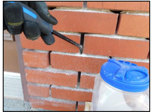
(Soft mortar) Soft and sandy mortar noted on the exterior bricks in various areas around the building. This is often caused due to presence of humidity over time. This condition can absorb more humidity causing further settlement and cracks over time. It is recommended to consult with a qualified masonry for further evaluation and proper corrections along with an accurate estimate of all associated costs before the signing at the notary.
