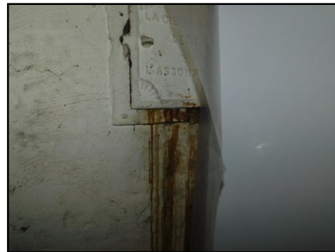
Infiltration from chimney cleanout, Recommend correction in this area
