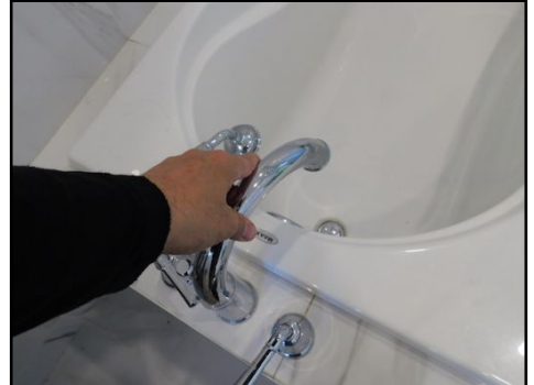
Plumbing fixture: - Loose bathtub faucet (No leaks noted). - Adjustment and application of silicone required to prevent water infiltration.
