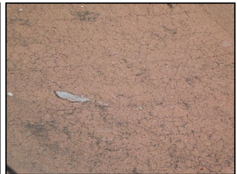
Evidence of patched repairs observed in a few areas (higher rooftop) and appears to be nearing/at the end of its lifecycle due to deterioration and cracks observed.
