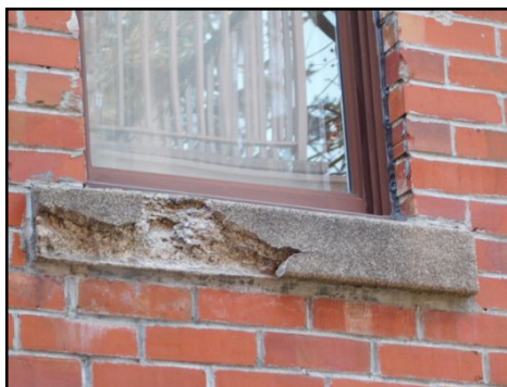
Some sill plates in need of repair/replacement (damaged/broken off) to prevent water infiltration and further damages.
