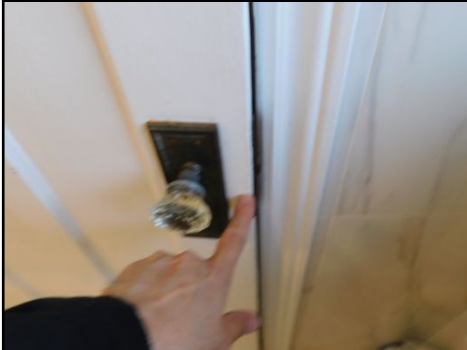
Bathroom door does not latch, adjustment needed
