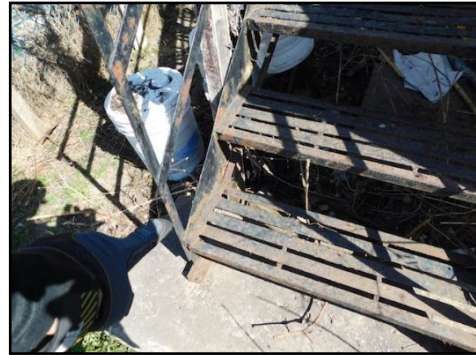
Loose area, safety hazard
