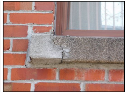
Some sill plates in need of repair/replacement (cracked, damaged/broken off) to prevent water infiltration and further damages.
