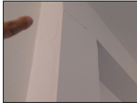
Walls and ceilings: Drywall/plaster, evidence of stress cracks in areas.
