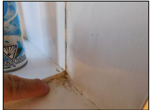
Walls and ceilings: Drywall. Previous signs of water damage/infiltration observed on the window sill sill. No moisture detected at the time of inspection. Verified with a moisture meter.
