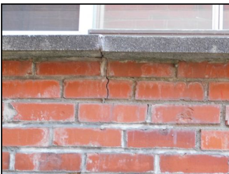
(Openings at the edges of the sill joints) Cracks/openings observed at the edges of the sill joints. This condition can lead to water infiltration and deteriorate the masonry materials below the windows in a faster speed. Repairs and corrections required on a regular basis to prevent degradation and spalling.
