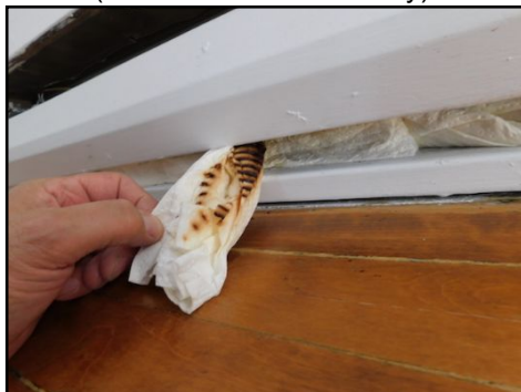
Electrical: One of the bedroom heaters had paper towels placed in the opening. Part of the paper towels were burnt. Serious fire hazard. This should be removed immediately.
