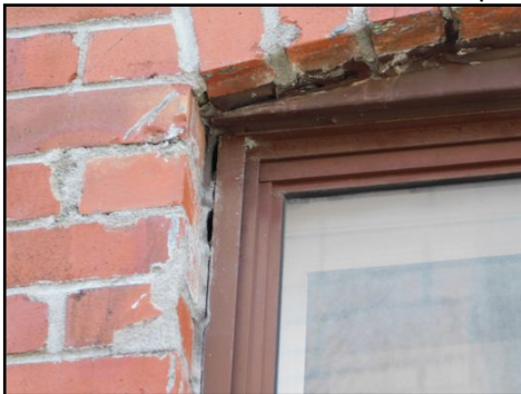
Important caulking needed, there are areas which need immediate repairs to prevent water infiltration, a caulking specialist should be contacted.
