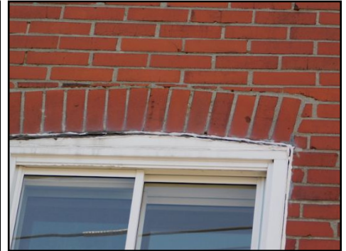
Examples of caulk needed around the house
