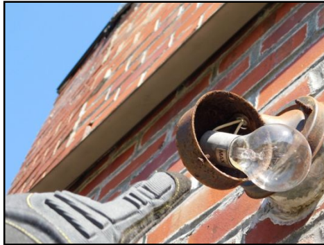
To be repaired, safety hazard
