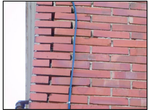
Major repointing needed in multiple areas around the building
