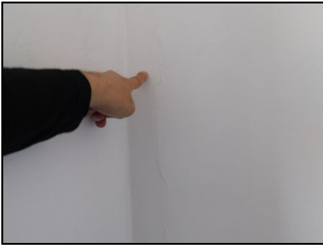
Walls and ceilings: Drywall/plaster, evidence of minor stress cracks.
