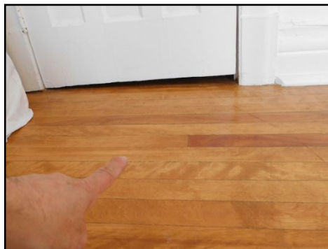
Floors: Sloping/central compression observed. See structure section for more info.
