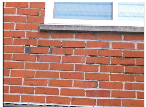
(Soft mortar) Soft and sandy mortar noted on the exterior bricks in various areas around the building. This is often caused due to presence of humidity over time. This condition can absorb more humidity causing further settlement and cracks over time. It is recommended to consult with a qualified masonry for further evaluation and proper corrections along with an accurate estimate of all associated costs before the signing at the notary.
