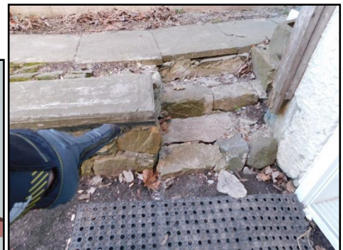
Loose steps/stones observed, by the side walkway. This is a trip/safety hazard. Corrections needed to enhance safety.
