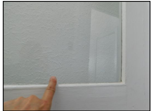
Door over stairs does not have tempered safety glass, this is a safety hazard.
