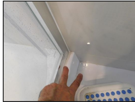
Standing shower and surrounding: Prefabricated fiberglass. Leaks noted (on both edges of the shower surrounding) at the time of the inspection. Repair required to prevent water damage.
