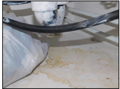
Previous water stains under the sink area
