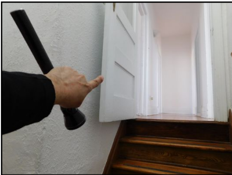
The door opens outward (over the stairs). This is considered a trip hazard and it should be corrected to be opened outward. Corrections recommended to enhance safety.
