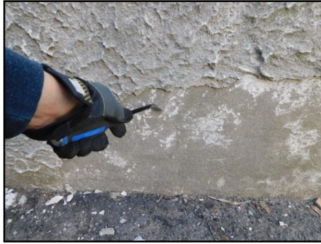
Minor foundation crack
