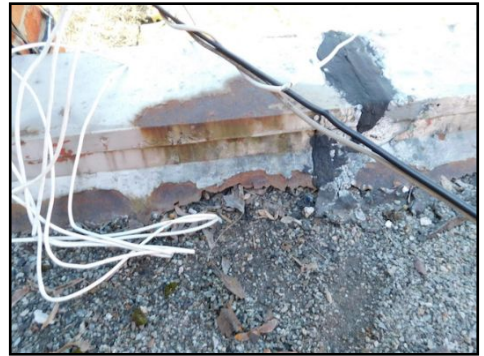
Corrosion, deterioration, openings and poor condition of the caulking was noted on the flashing. This condition can easily lead to water infiltration within the walls. Corrections required by a qualified roofing contractor.
