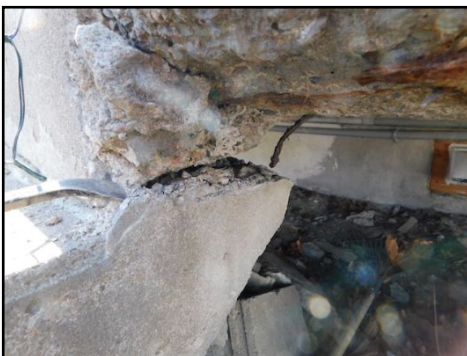
Concrete deterioration and rusted rebar is exposed. Possibility of detaching concrete stairs from the concrete balcony. Further verification is required and repair as needed.
