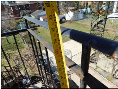
Guard rails height are too low for today's safety standards. Although this is typical based on the age of the construction, it is considered a safety hazard and it should be corrected to enhance safety.
