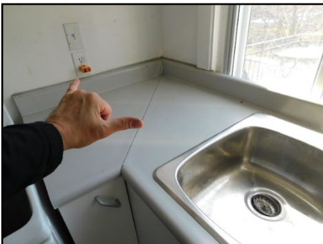
Electrical: - Outlet next to the sink not protected with GFCI. This is a safety hazard and it should be corrected to enhance safety.
