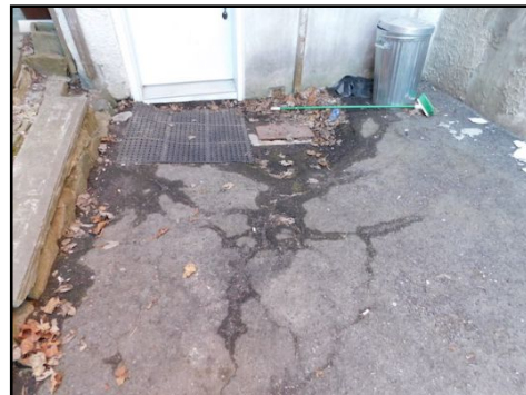
There was some degree of cracking and/or damage present to the driveway asphalt surface. If a concern, have an asphalt paving company or other qualified person to evaluate for repair.
