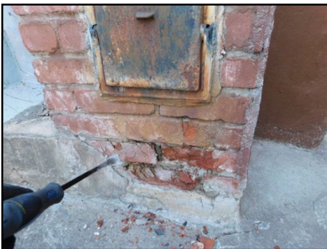
(Brick spalling) Visible brick spalling noted. This is mostly associated with presence of water/moisture behind the bricks. Further investigation and proper corrections is recommended to prevent further damages.
