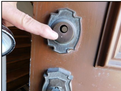
A hole observed in the keyhole area. Repair recommended (#5412)
