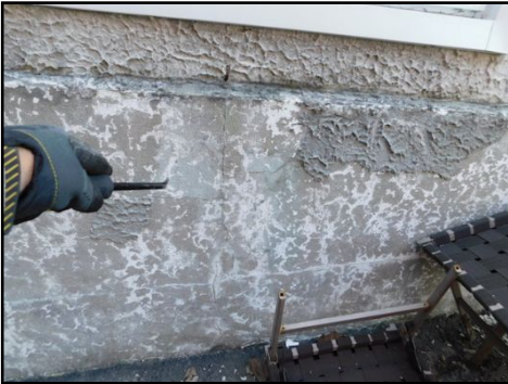
Minor foundation crack observed
