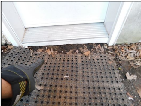
The basement door sill is too close to ground, water could infiltrate, a distance of at least 4 inches from ground is required.
