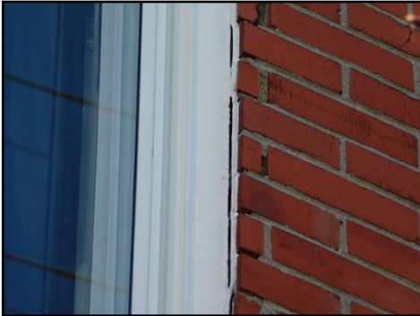
Important caulking needed, there are areas which need immediate repairs to prevent water infiltration, a caulking specialist should be contacted.
