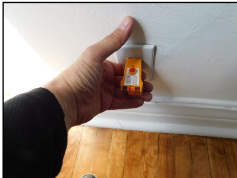
Electrical: Outlets are NOT grounded (Also see main electricity).
