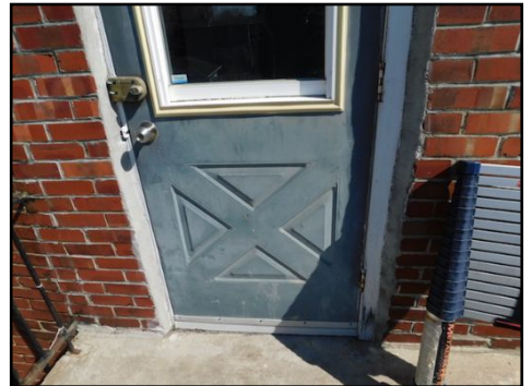
Rear upper balcony door: Opening outward (exterior) with hinges installed on the exterior portion. This condition may be a concern due to the fact that it may be removed. (Security concern)
