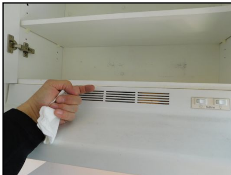
Hood Fan does not vent to the exterior. Recommend having it vent to the exterior.
