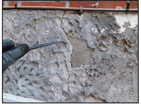
Foundation crack to be verified by foundation specialist and repair as needed
