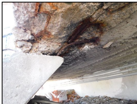
Concrete deterioration and rusted rebar is exposed. Possibility of detaching concrete stairs from the concrete balcony. Further verification is required and repair as needed.
