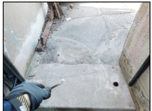
Uneven walkways were observed, this is a trip hazard
