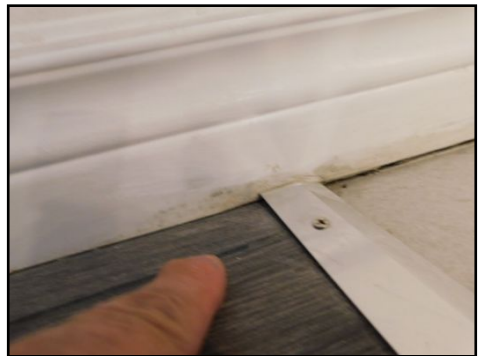
Walls and ceilings: There appears to be Mold like substance observed on the baseboards where it was not properly painted. Cannot confirm this is Mold, however, there were a few areas like this that was observed where it was not properly painted. If this is a concern, recommend further verification behind the baseboards.
