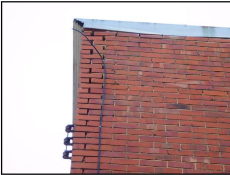
(Brick detachment) Visible brick detachment, and some appear to be bowing outwards was noted on upper portion of the building. This is often associated with water infiltration and freezing and is usually caused by improper flashing of the roof. Repairs and corrections required by a qualified contractor to prevent further damages.
