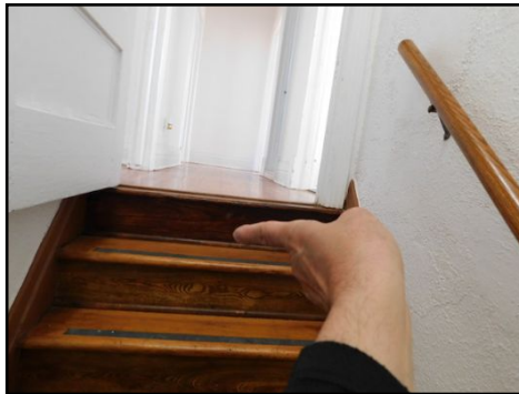
Floor levelling: Sloping/central compression observed.
