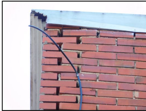
Risk of water entering building/weakened structure/chance of structural movement.
