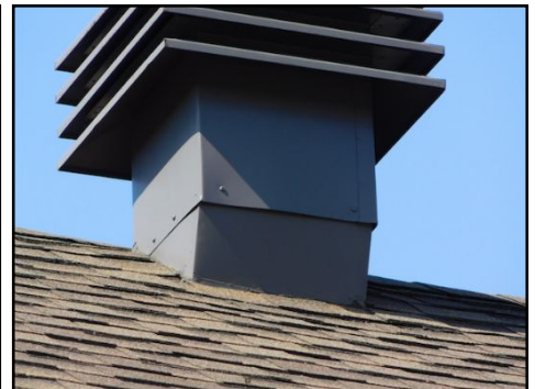
(Flashing installed under shingles) The flashing of the roof penetrations are installed under the shingles. (The lower portion of the flashing should be installed over the shingles. This will allow the water slide on the surface). Application of proper caulking and close monitoring for any signs of leaks is recommended. (Part of regular maintenance when flashing installed under shingles)
