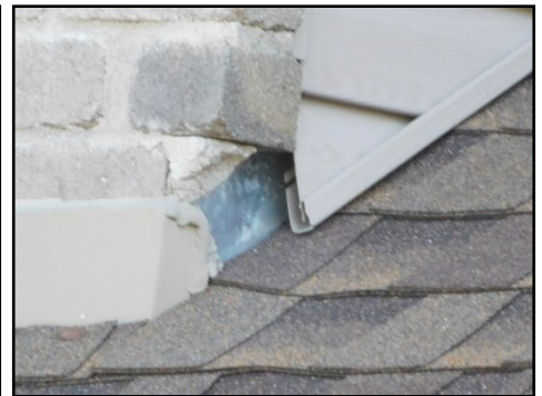
It appears that there may be a small brick or flashing missing just above the garage roof area. This is a risk of water infiltration. Repair is required to prevent possible water intrusion.
