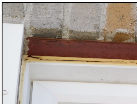
Lintels above the windows (and door) are not painted. Application of exterior paint for extra protection to prevent rusting is recommended.
