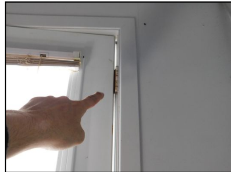
Side door hinge is loose and needs to be adjusted. (As seen from inside the garage)
