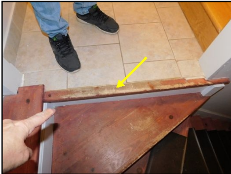
Top step is slightly and is a safety hazard. Repair needed to enhance safety
