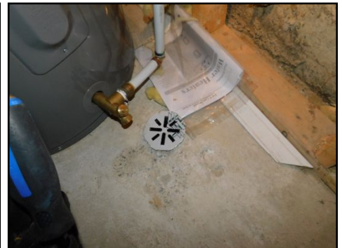
The floor drain is located in the basement, next to the hot water tank, however the efficiency of the floor drain is not within the scope of this inspection. (Floor drain may dry out over time and letting sewer smell entering the building. Adding water on regular basis is recommended)
