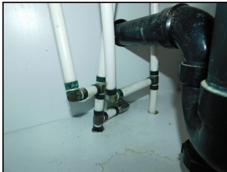
Corrosion observed at some of the fittings, no leaks visible at time of inspection. Recommend review by a licensed plumber for repair or replacement, as necessary, prior to close.
