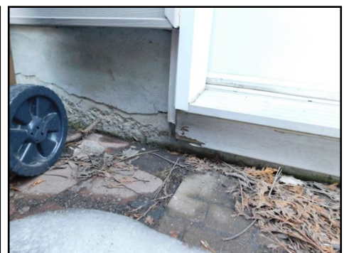
Cement parge coat is flaking/deteriorated in some areas. Recommend review for repair as necessary.
