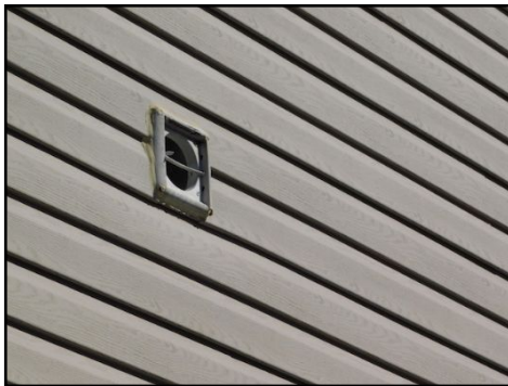
All cracks and openings on exterior coverings should be sealed and repaired to prevent water infiltration and further damages. (Including the openings for the bathroom vents. Risk of wildlife entering). A grill/cover is required
