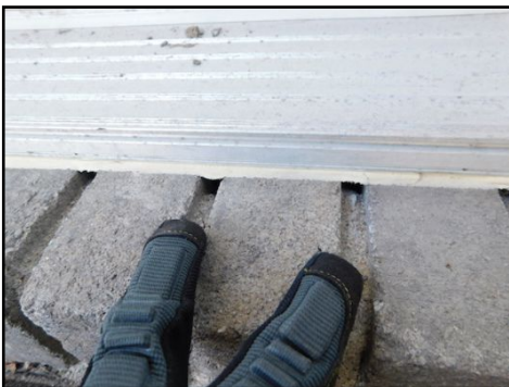
Minor caulking needed around the house, touch up the areas which may be vulnerable to water infiltrations.
