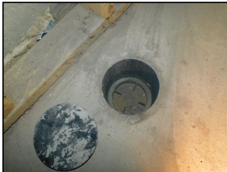
Backwater valve located in the basement, (visible during inspection).
