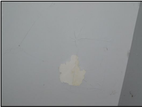
Evidence of past water penetration observed, however it is dry at the time of the inspection.
