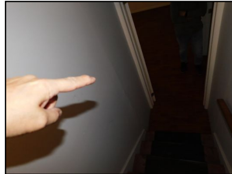
Missing three way switch for proper lighting. Corrections recommended to enhance safety.
