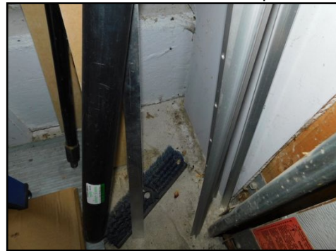
Evidence of past water penetration observed, however it is dry at the time of the inspection.
