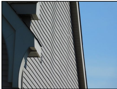
Minor warping observed, this is sometimes due to tight installation and previous house settlement
