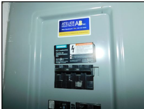
The main electrical panel has a maximum capacity of 150 amps
