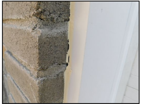
Examples of caulk needed around the house
