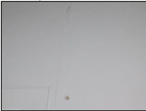
Minor tension crack, repair as needed
