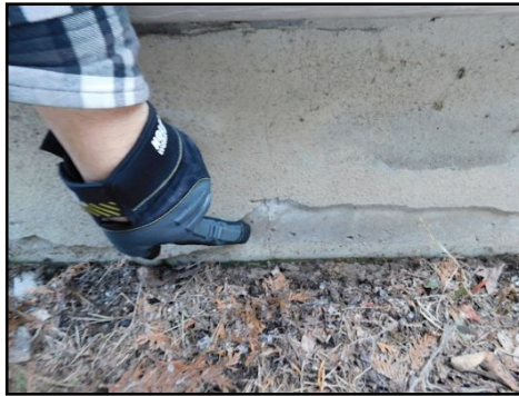
Minor foundation crack
