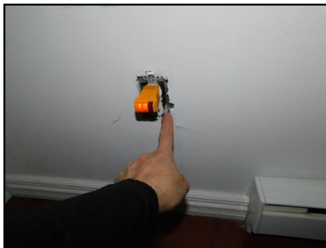
Missing faceplate, this is a safety hazard. Installation needed to enhance safety
