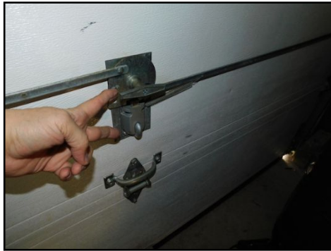
Minor correction needed with the knob, to spring open
