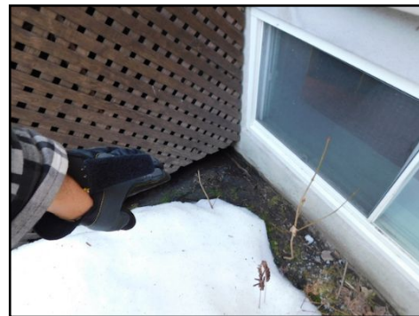
Negative slope in areas
