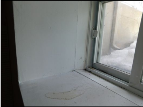
Previous water stains and water damage observed on the windowsill and above the window. No moisture detected. Close monitoring is recommended for any possible further infiltration. This may also be due to lack of caulking on the exterior.
