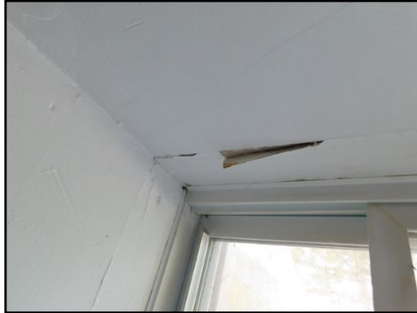
Previous water stains and water damage observed on the windowsill and above the window. No moisture detected. Close monitoring is recommended for any possible further infiltration. This may also be due to lack of caulking on the exterior.
