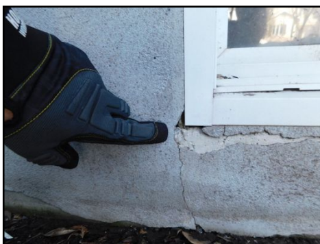
(With cracks) Presence of minor/important cracks were observed in areas around the foundation. They require further verification by a certified foundation specialist, and to be repaired, if needed
