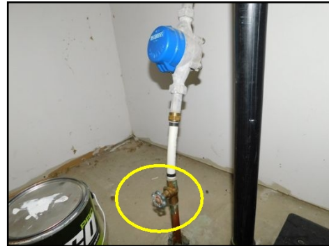
Usable at the time of the inspection, however these types of valve can leak over time. Recommend replacing with a lever type valve.
