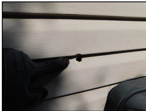
All cracks and openings on exterior coverings should be sealed and repaired to prevent water infiltration and further damages. (Including the openings for the bathroom vents. Risk of wildlife entering). A grill/cover is required
