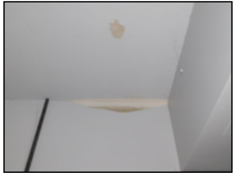
Evidence of past water penetration observed, however it is dry at the time of the inspection.
