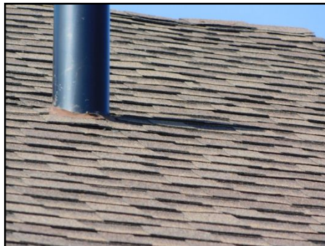
(Flashing installed under shingles) The flashing of the roof penetrations are installed under the shingles. (The lower portion of the flashing should be installed over the shingles. This will allow the water slide on the surface). Application of proper caulking and close monitoring for any signs of leaks is recommended. (Part of regular maintenance when flashing installed under shingles)
