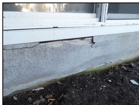
Cement parge coat is flaking/deteriorated in some areas. Recommend review for repair as necessary.
