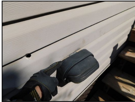
Examples of caulk needed around the house
