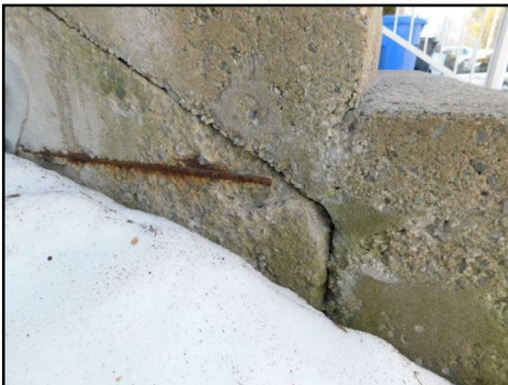
Due to the deterioration of the concrete on the side, there is one rebar that is exposed. Exposed and rusted rebar's can weaken the concrete around the area. Repair as needed. Contact a certified cement finisher.
