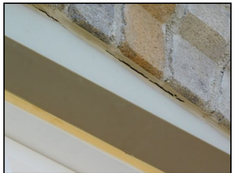
Examples of caulk needed around the house
