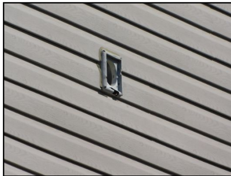
All cracks and openings on exterior coverings should be sealed and repaired to prevent water infiltration and further damages. (Including the openings for the bathroom vents. Risk of wildlife entering). A grill/cover is required
