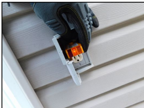
Exterior outlets are not protected with GFCI. Installation recommended for today's standards.
