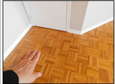
Minor sloping/central compression observed
