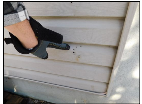
All cracks and openings on exterior coverings should be sealed and repaired to prevent water infiltration and further damages. (Including the openings for the bathroom vents. Risk of wildlife entering). A grill/cover is required
