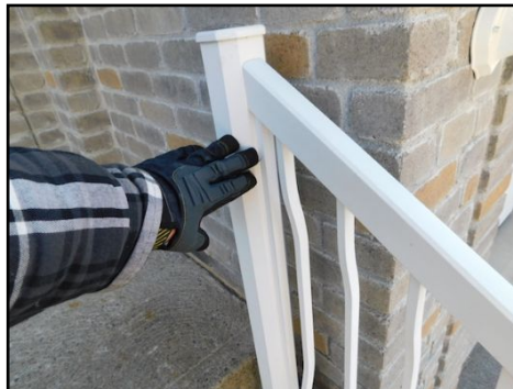
Loose handrail noted on the main stairs. This is considered a safety hazard and it should be corrected to enhance safety.
