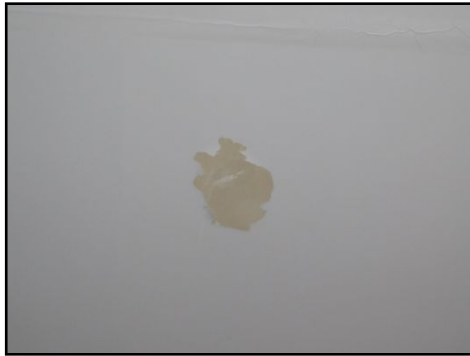
Evidence of past water penetration observed, however it is dry at the time of the inspection.
