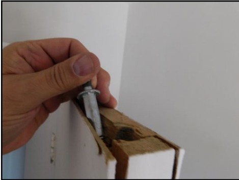
Physical damages noted. Repair / replacement recommended as needed.
