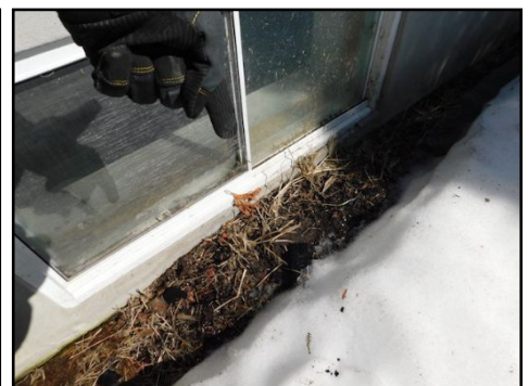
Missing window wells noted on the basement windows. Installation recommended. (Window wells are required on all windows placed within 6 inches to the ground level to prevent snow accumulation and water infiltration).
