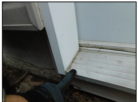
Examples of caulk needed around the house
