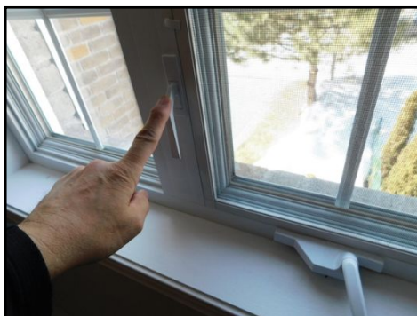
Minor adjustment needed with latches in master bedroom
