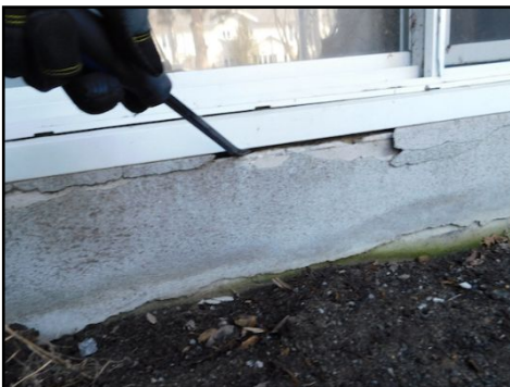
Minor caulking needed around the house, touch up the areas which may be vulnerable to water infiltration.
