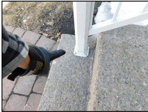
Loose handrail noted on the main stairs. This is considered a safety hazard and it should be corrected to enhance safety.
