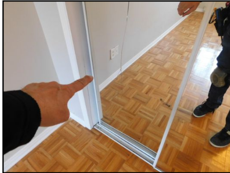
Cracked sliding mirrored door. Safety hazard. Replacement required.
